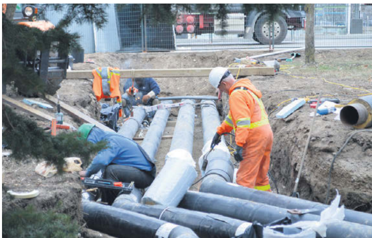
Workers install pipes at Guelph's Sleeman Centre, which will be part of North America's first city-wide district energy network. In addition to bringing massive savings in fuel, equipment and maintenance costs, this initiative will lead to a much smaller environmental footprint. SUPPLIED
